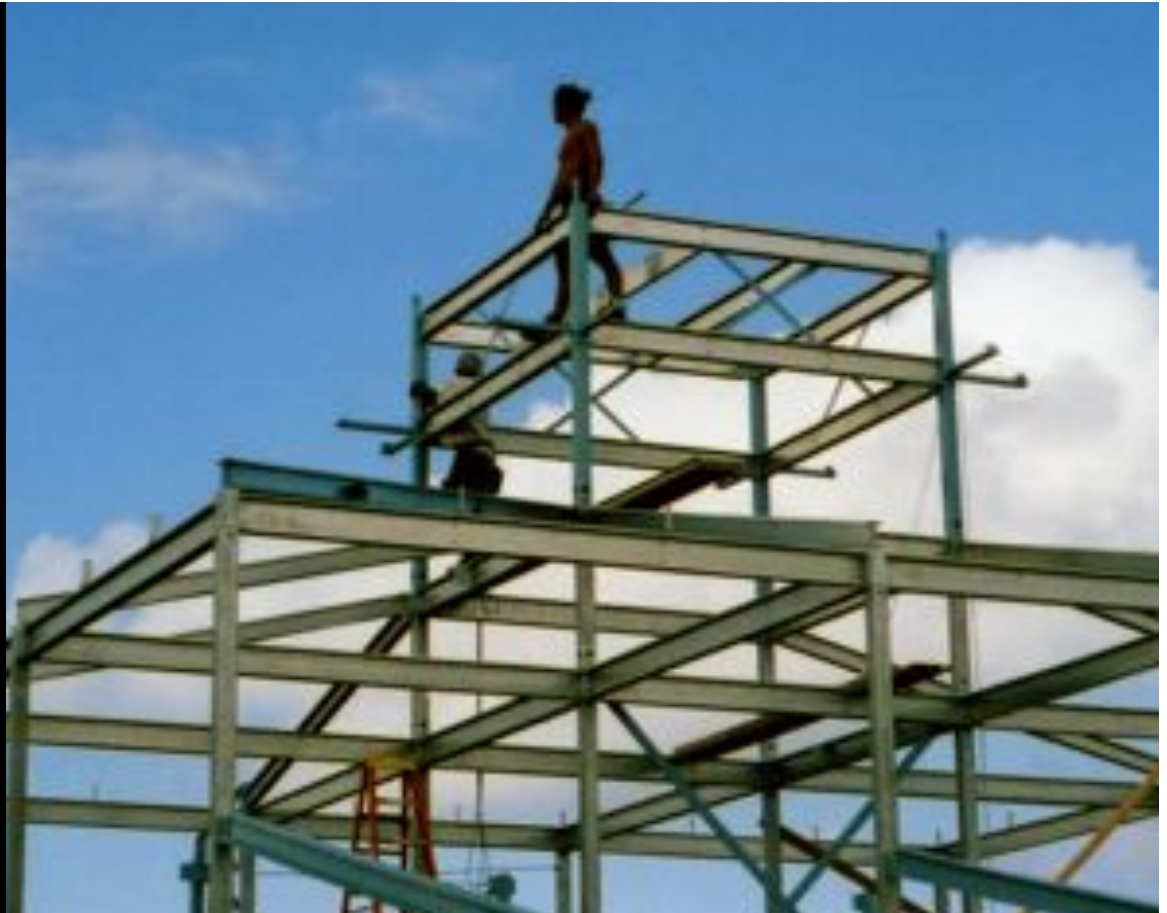
Workers pause to look at whales during frame assembly of the Honomu House in Hawaii.
